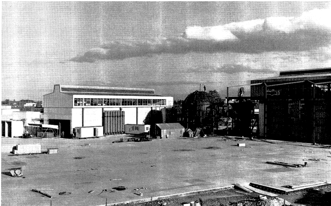
'A laboratory is never finished . . .' A recent view of part of the new East experimental area, still under construction for the CERN proton synchrotron. The end of the building to house the 1.5-m British Hydrogen Bubble Chamber and the CERN 2-m hydrogen chamber can be seen on the right, with the hydrogen safety sphere between it and the compressor building. The safety sphere is designed to receive the hydrogen from either chamber in the event of an accident.
